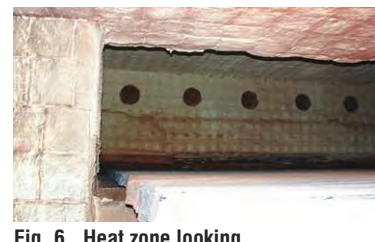
Fig. 6. Heat zone looking into soak zone
