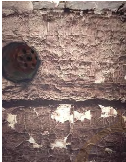
Fig. 11. Burner wall with minimal damage
