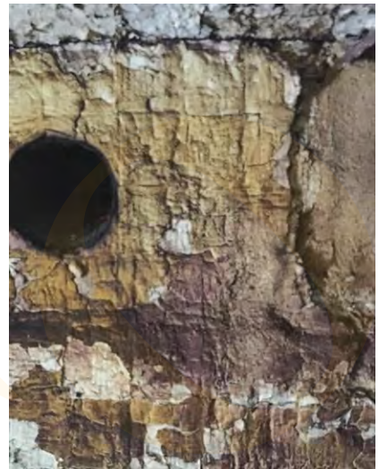
Fig. 12. Damaged burner wall
